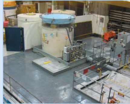
A Demineralizer was installed on Unit 1 to remove impurities from the water in the spent fuel pool.
